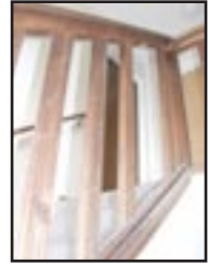
Interior or common area stairways frequently fail inspection due to missing vertical rails.
